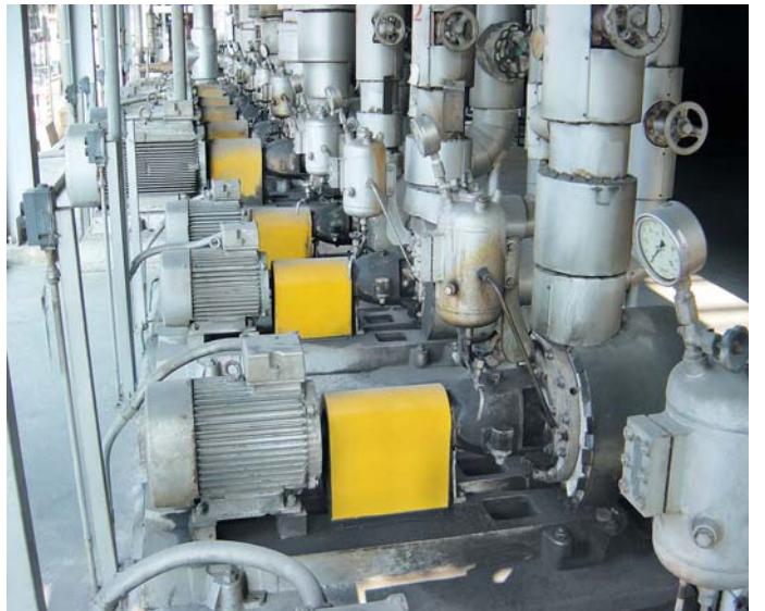
Type NCL with tandem bellows seal (N9). Liquid: Thermal oil, 330°C (626°F).
