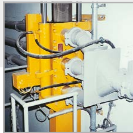
Gate valves for there different delivery lines
