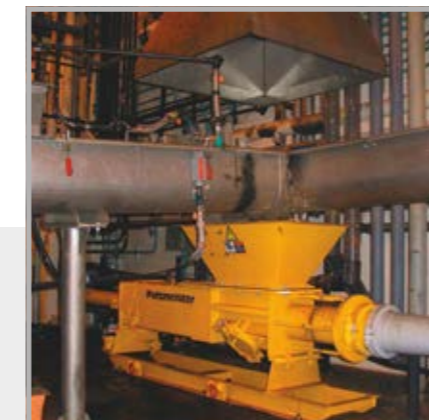
Pumping screenings (Coney Island, New York)
