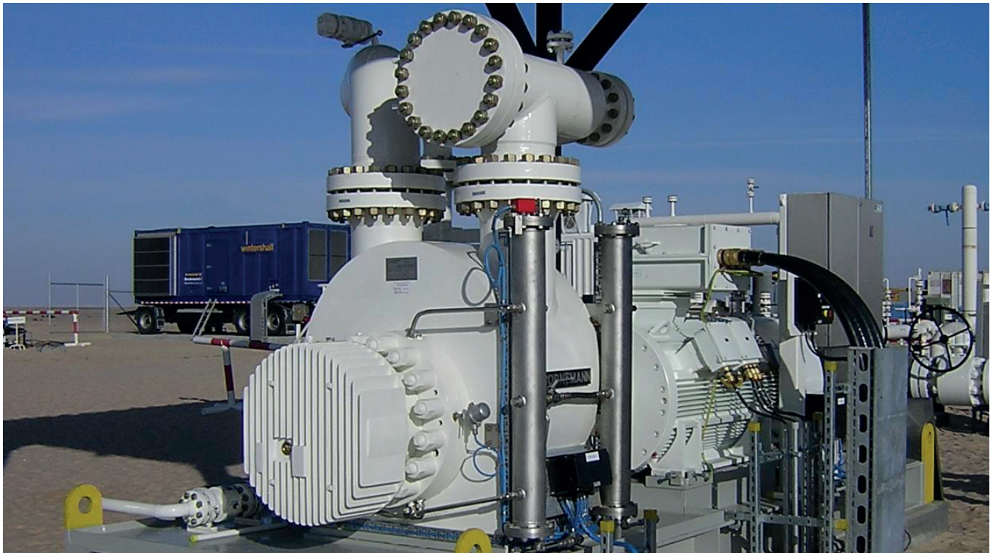
Multiphase „Boosting in Libya“
